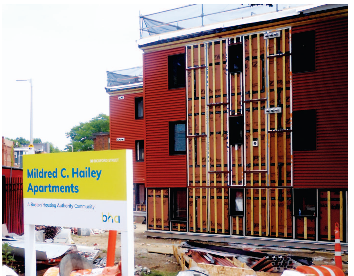
A view of the construction at 170 Heath Street at Walden Street for the new apartments at Mildred C. Hailey complex.
